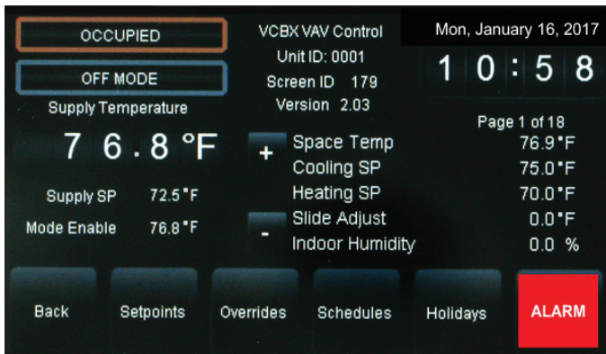
Figure 20: Controller Status Screen (VCC-X Shown)
